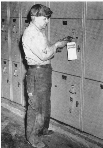
Louis Kemp, electrician, places a Danger Tag on a control before he checks a piece of electrical equipment.
